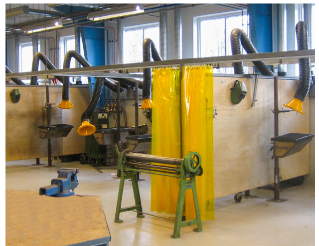
Wing arms Ø160mm 3m installed at technical school. Including automatic control devices for automatic start/stop of fan and motor damper.
